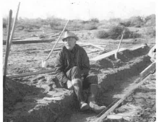
Tom Roberts takes a break as the footings for the South wall are made.
