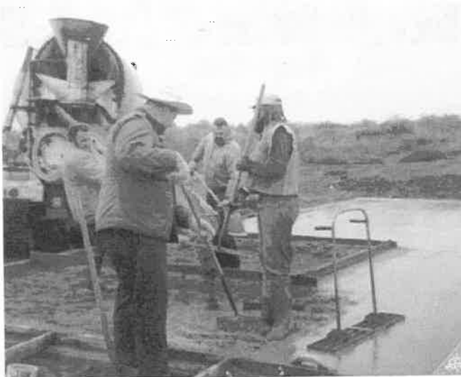
Pouring concrete floors. Facing the camera is Virgil DeChand, facing away is Marvin Haws.
