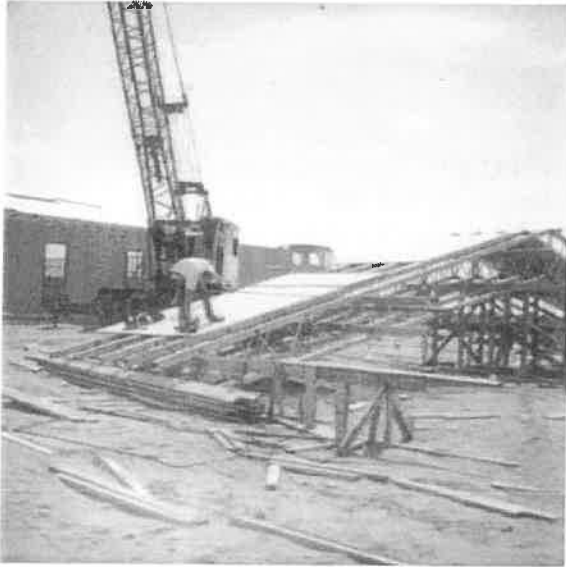
Preparing sections of the roof trusses on ground before lifting by crane into place.
