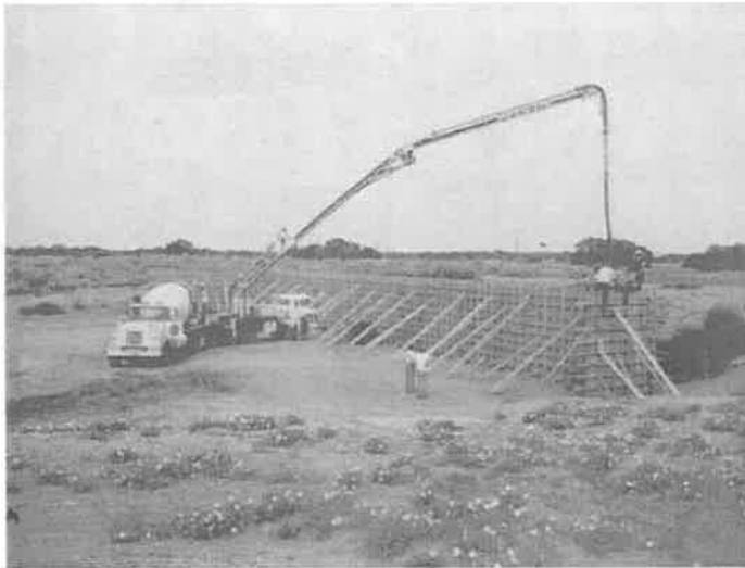
Pouring the North wall. All one continuous pour made in one day.
